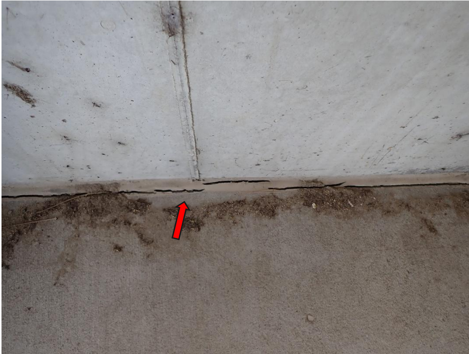
Photo 8. Representative failed cove sealant at wall perimeter (Seminary shown; others similar).
