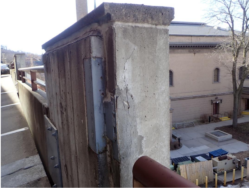
Photo 46. Representative delaminated area at precast concrete facade panel and coping piece.
