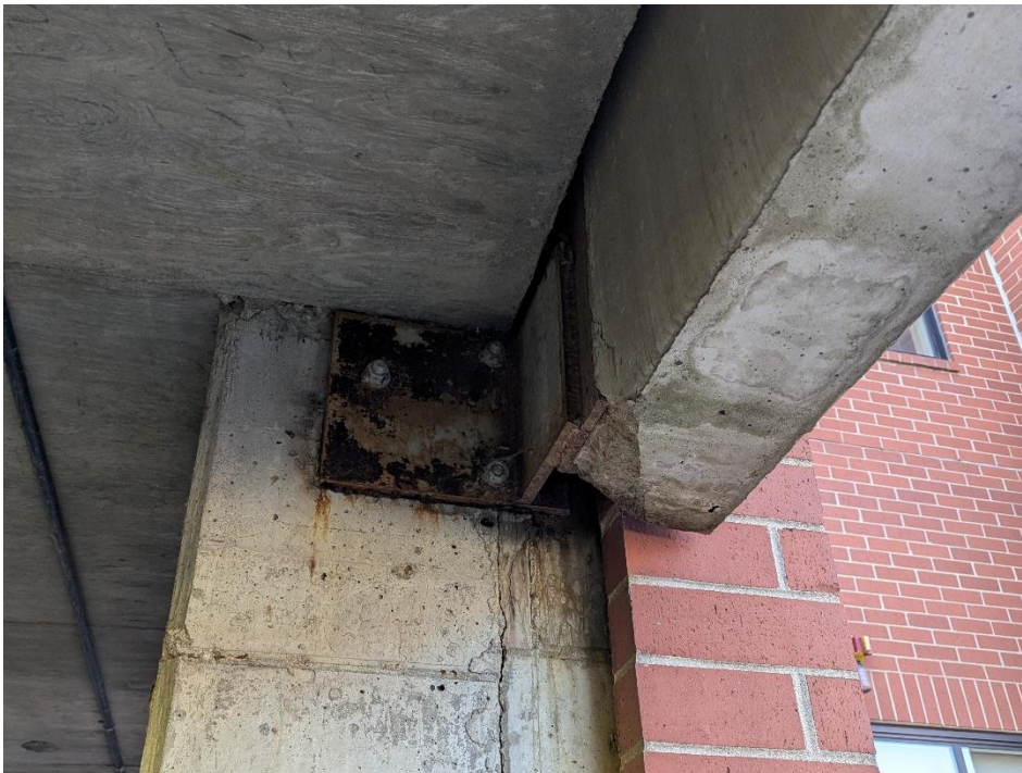
Photo 55. Representative peeling paint and surface corrosion on steel connections for the precast facade panels.
