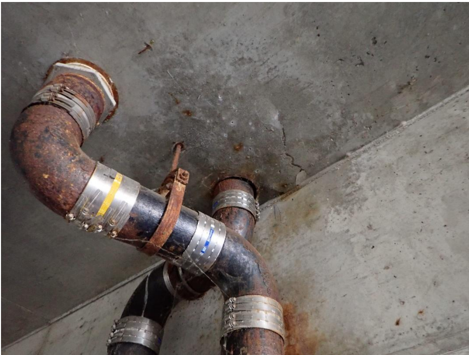
Photo 27. Cracked drain pipe at the southwest corner of the Ground Level.
