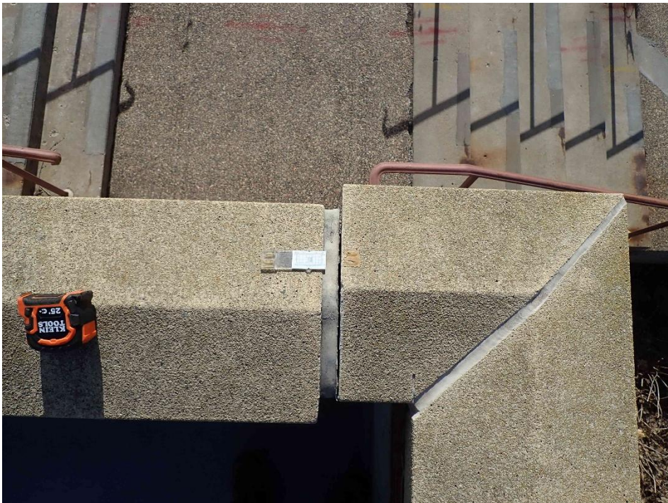
Photo 25. Close-up view of shifted facade walls at the southwest corner of the ramp, looking down.
