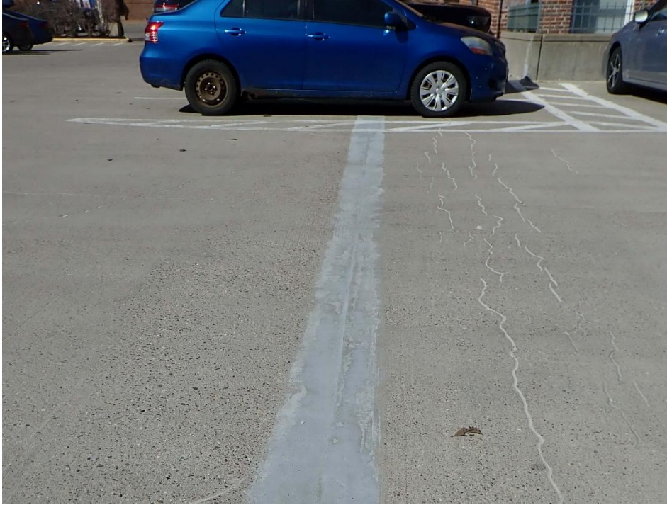
Photo 10. Representative worn waterproofing membrane at construction joint (Studebaker shown; others similar).
