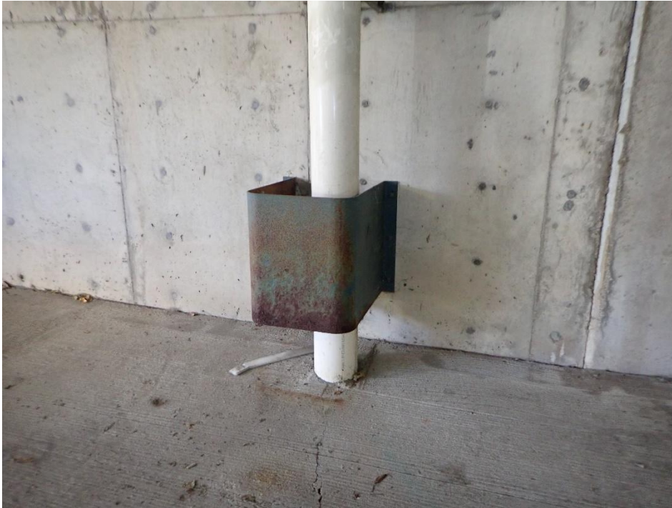
Photo 36. Representative peeling paint and surface corrosion on steel pipe guard at the Lower Level.
