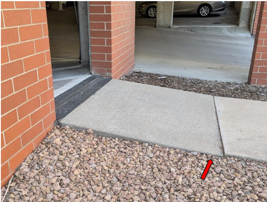
Photo 62. Settled sidewalk panel at one corner at the pedestrian entrance at the southwest street level (Level B).
