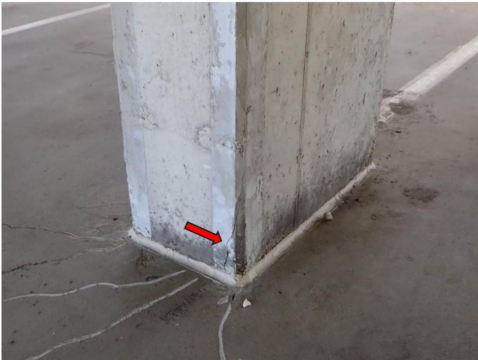
Photo 5. Representative delaminated area at concrete column (Seminary shown, others similar).
