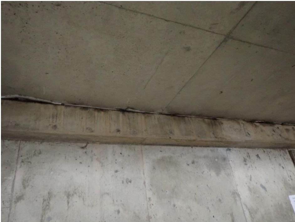
Photo 29. View beneath winged expansion joint at the west entrance/exit on the Main Street Level. Water stains are evidence of failed joint above.
