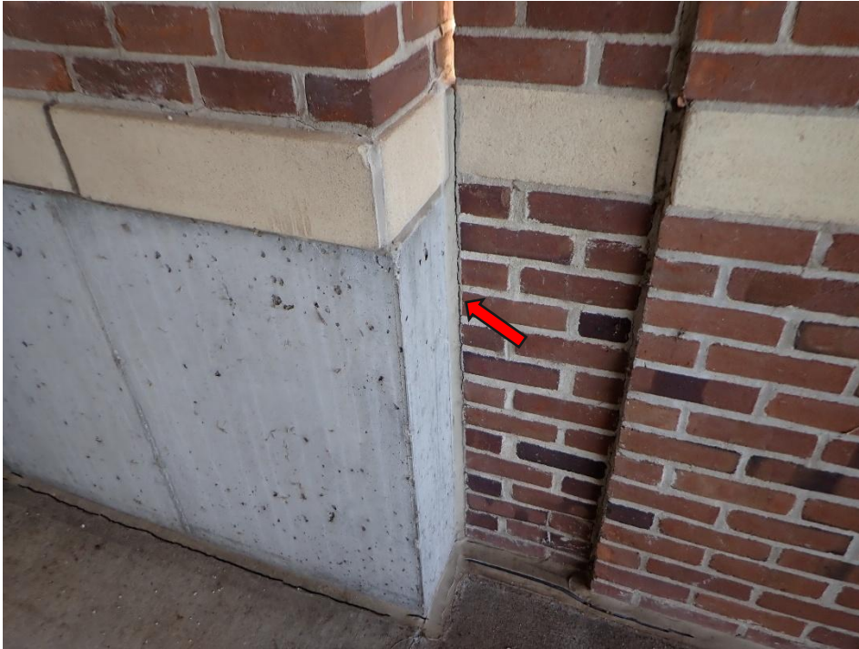
Photo 14. Failed sealant joint on the interior side of a precast panel on the Second (middle) Level.
