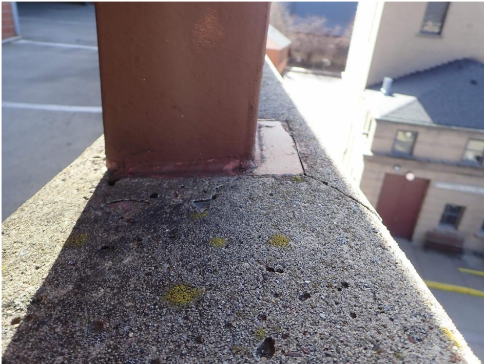
Photo 47. Representative delaminated area at precast concrete facade panel.
