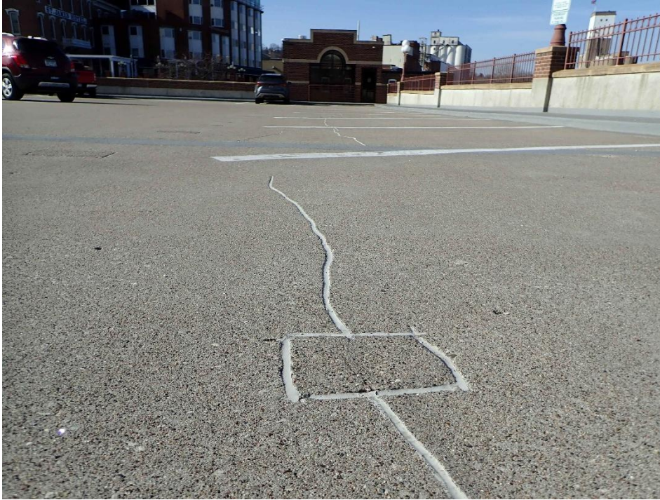
Photo 6. Representative failed sealant in previously routed and sealed floor cracks (Seminary shown; others similar).
