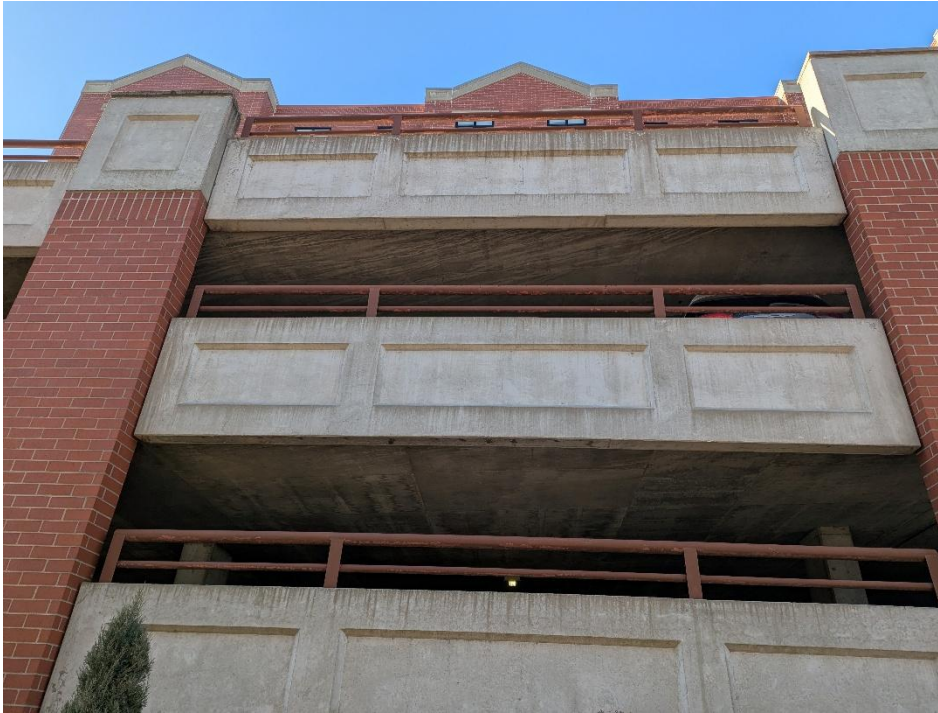
Photo 56. Representative peeling paint and surface corrosion on steel pedestrian railings at all facades.
