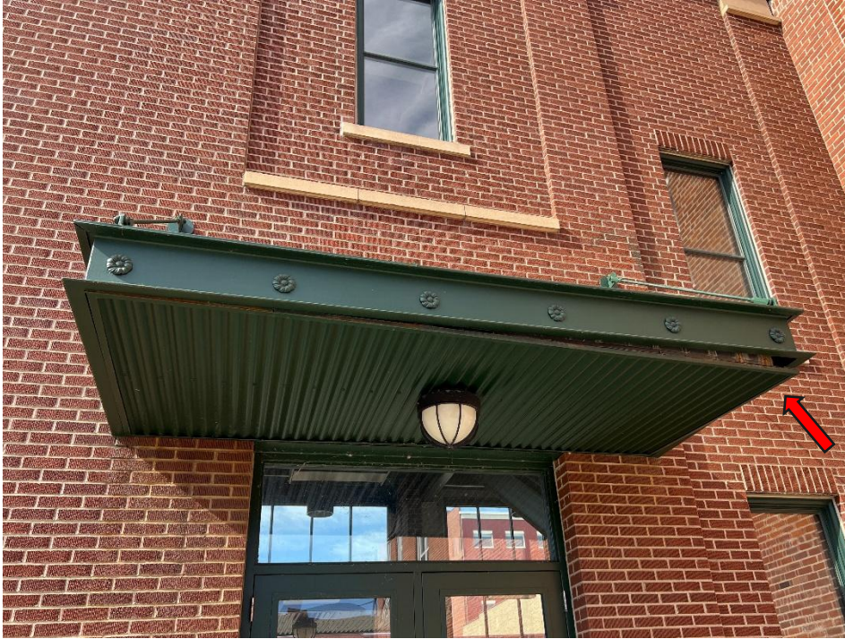
Photo 40. Displaced/loose corrugated metal soffit piece at one corner at the south side of the elevator tower awning.
