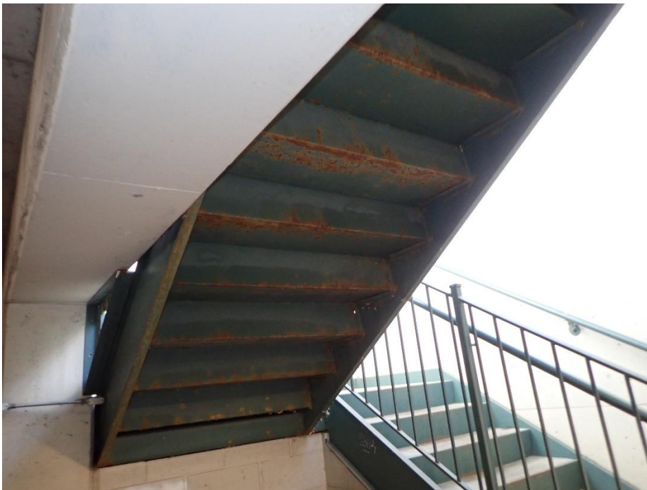
Photo 37. Representative peeling paint and surface corrosion on metal stair treads/pans, stringers, and railings in the west stair tower.
