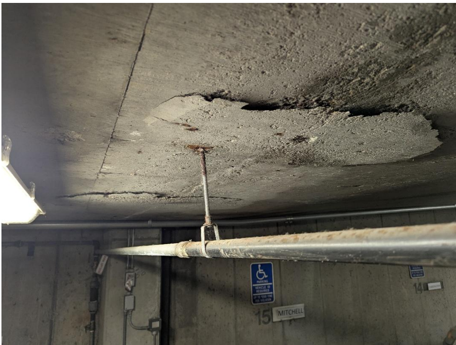
Photo 43. Representative pipe hanger at ceiling spall on Level A.
