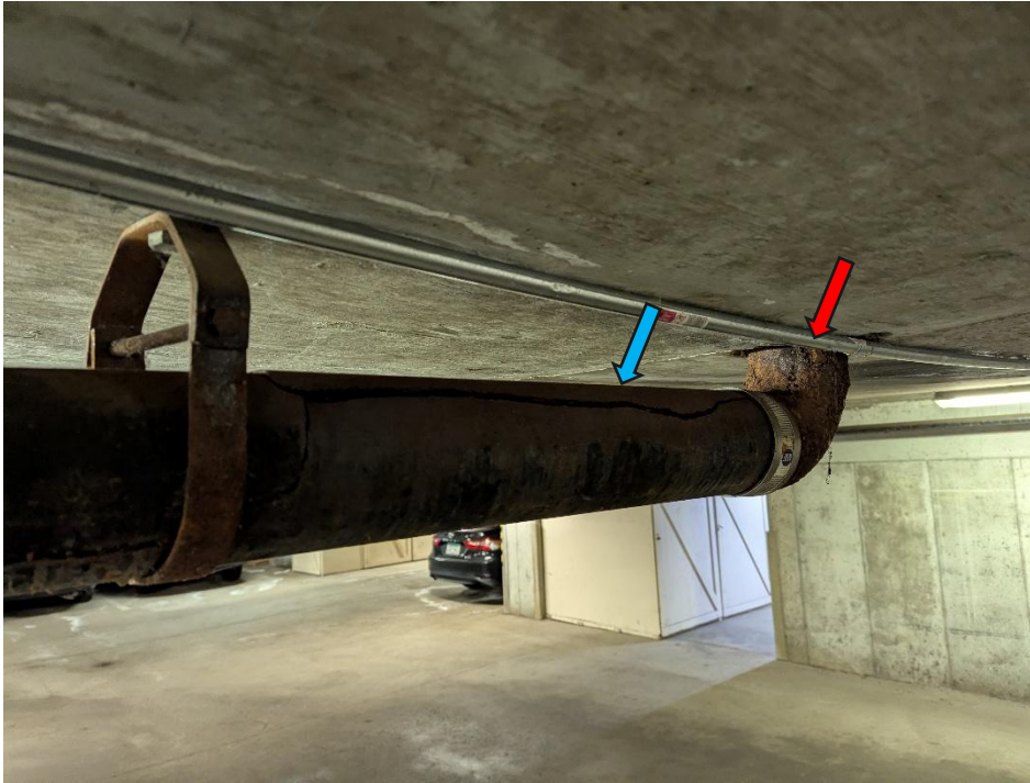
Photo 63. Corroded drain body (red arrow) and representative cracked section of pipe (blue arrow) on Level A.
