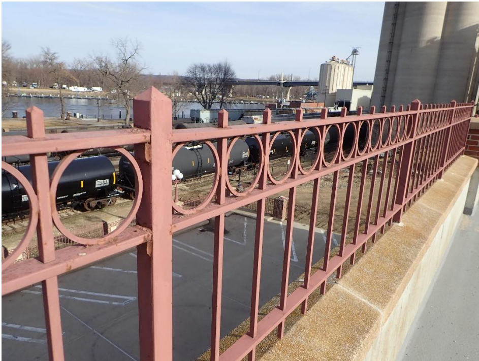
Photo 17. Representative peeling paint and surface corrosion on pedestrian railings, fencing, and light posts on the Plaza (top) and Ground (lowest) Levels.
