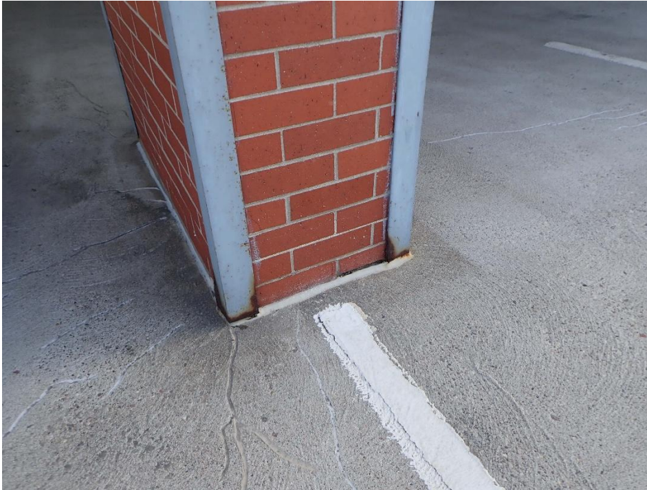
Photo 58. Representative peeling paint and surface corrosion on metal column corner guards on Level E.
