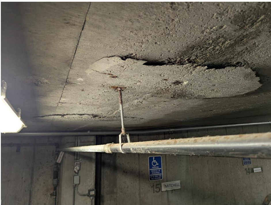
Photo 3. Representative delaminated area at concrete ceiling (Seminary shown, others similar).
