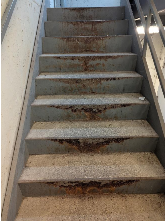
Photo 60. Representative peeling paint and surface corrosion on metal stair treads/pans, stringers, and railings.
