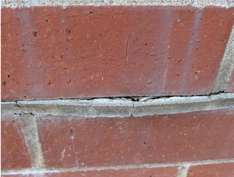
Photo 50. Representative cracked brick mortar joint.
