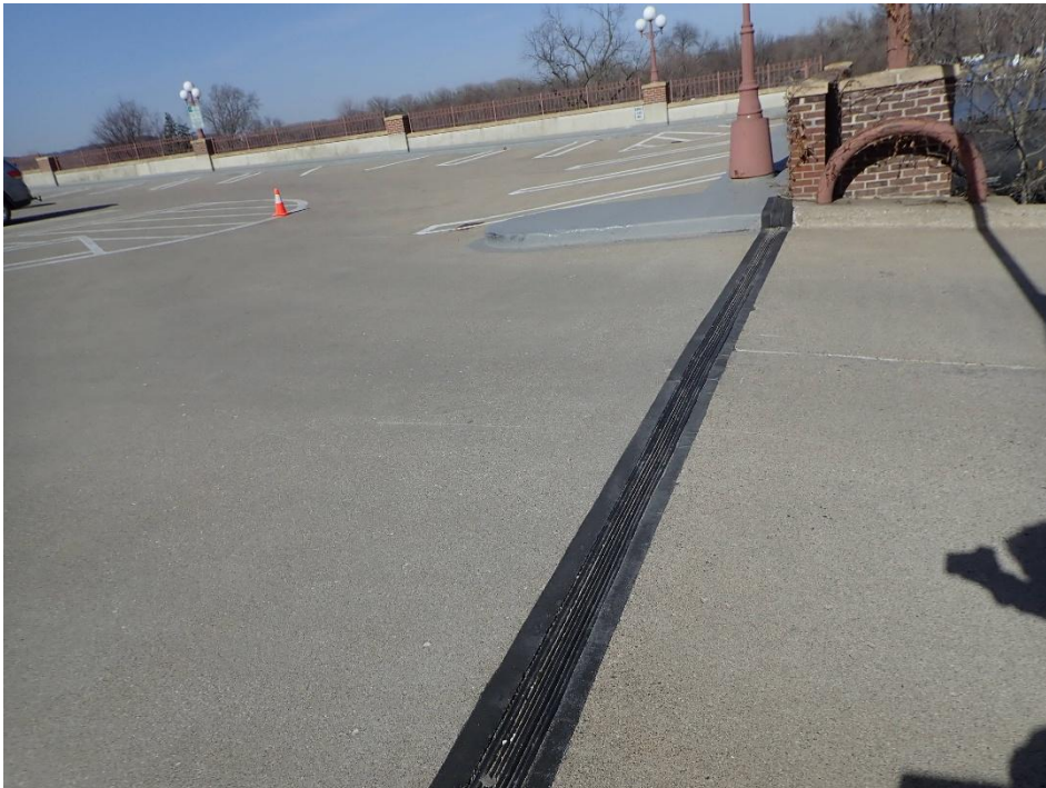
Photo 13. Overall view of winged expansion joint with isolated tears throughout at the entrance/exit of the Plaza (top) Level at the east side of the structure.
