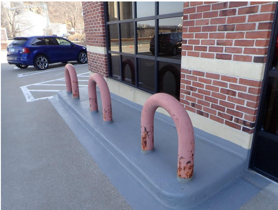
Photo 15. Representative peeling paint and surface corrosion on vehicle barriers (Top Level shown; Ground Level similar).
