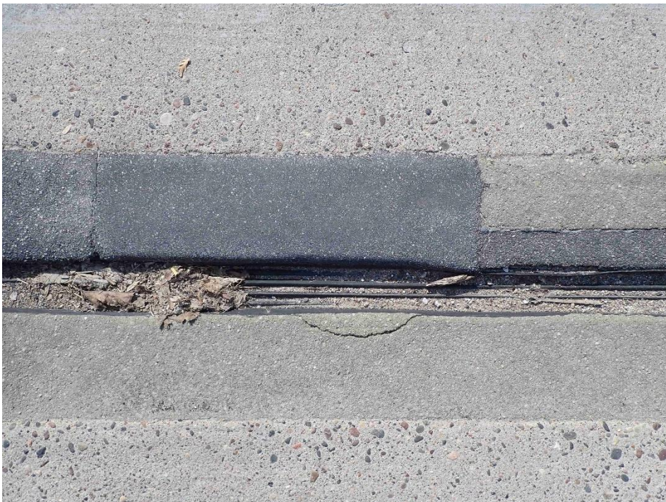
Photo 31. Representative cracked elastomeric header material throughout the winged expansion joint near the west-middle of the structure on the Main Street Level.
