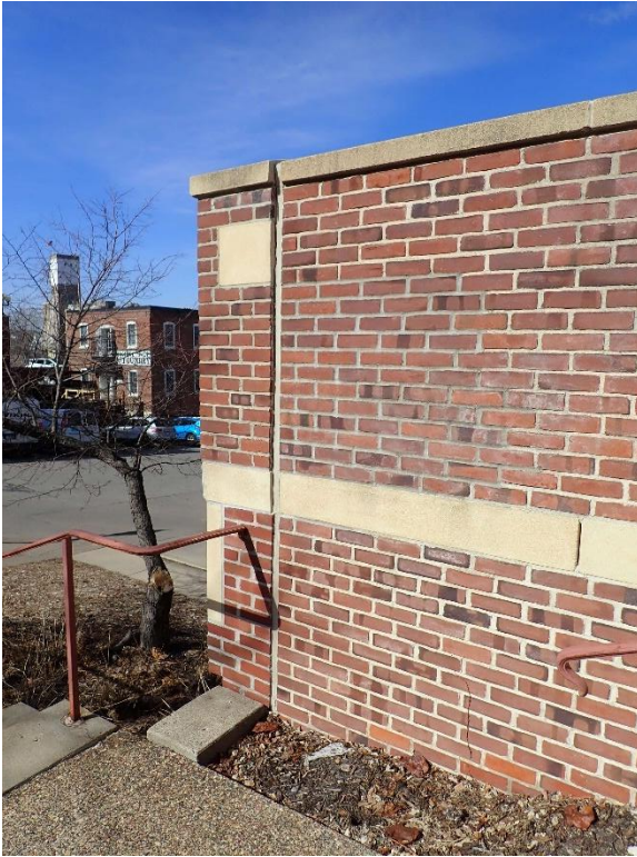
Photo 26. Overall view of shifted facade walls at the southwest corner of the ramp, looking north-northwest.
