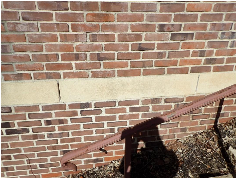
Photo 23. Representative open and weathered mortar joints in brick and precast facade.
