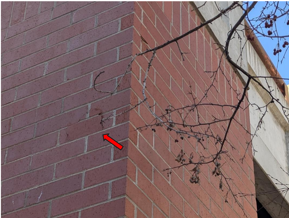
Photo 51. Representative cracked brick at isolated location on facade.
