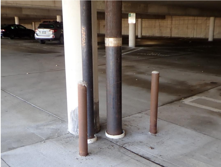
Photo 16. Representative unpainted bollards on Ground Level with surface corrosion.
