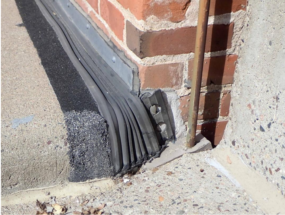
Photo 30. Representative failed end termination at winged expansion joint on the Main Street Level.
