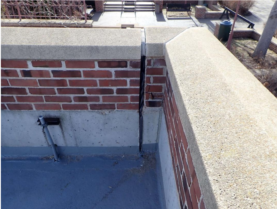
Photo 24. Overall view of shifted facade walls at the southwest corner of the ramp, looking south-southeast.
