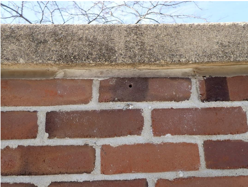
Photo 21. Representative location of weathered and cracked sealant in bed joint below coping piece.
