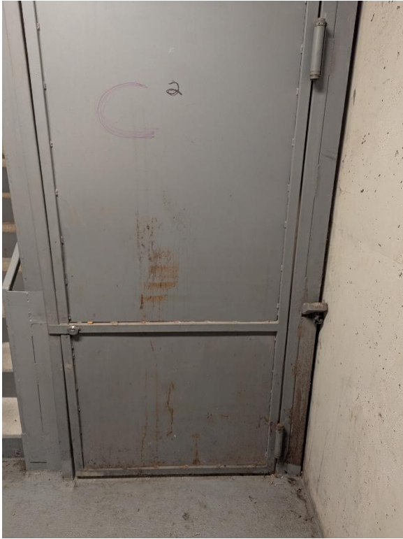
Photo 61. Representative peeling paint and surface corrosion on metal doors and frames.
