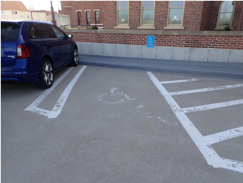
Photo 11. Representative worn traffic markings (Seminary shown; others similar).
