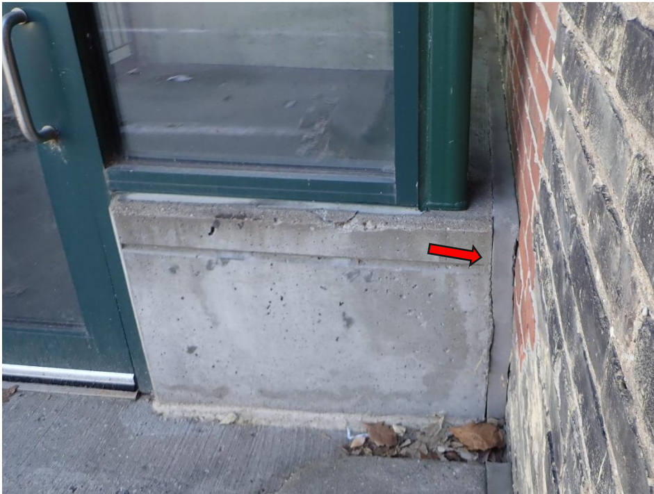
Photo 7. Representative failed foam adhered expansion joint (Studebaker shown; others similar).
