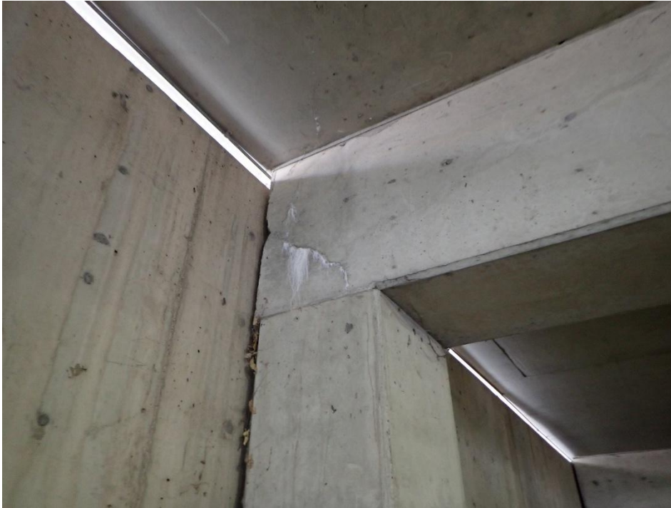
Photo 4. Representative delaminated area at concrete beam (Studebaker shown, others similar).
