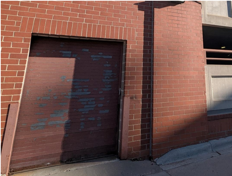
Photo 59. Representative peeling paint and surface corrosion on metal garage door and frame at the east end of the north alley on street level.
