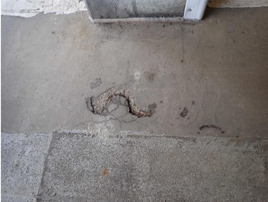
Photo 2. Representative delaminated area at concrete floor (Seminary shown, others similar).
