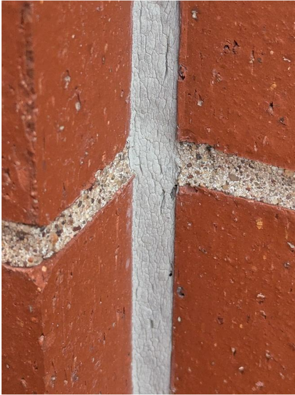
Photo 54. Representative failed sealant at brick control joint.
