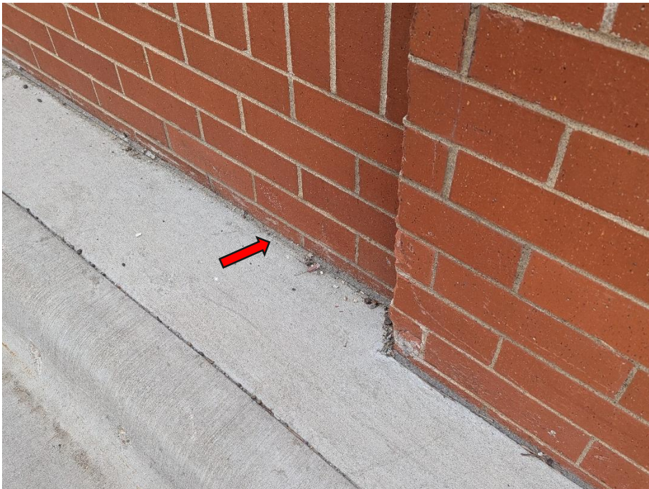
Photo 9. Representative view of missing cove sealant at entire perimeter of the Studebaker Main Street Level.
