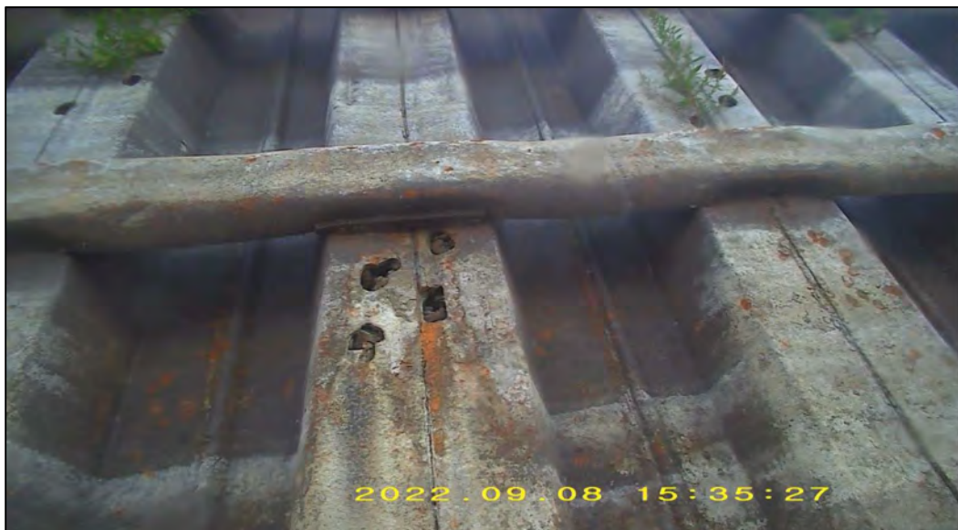
Figure 2: Holes in SSP at Old Timber Fender attachment Points
