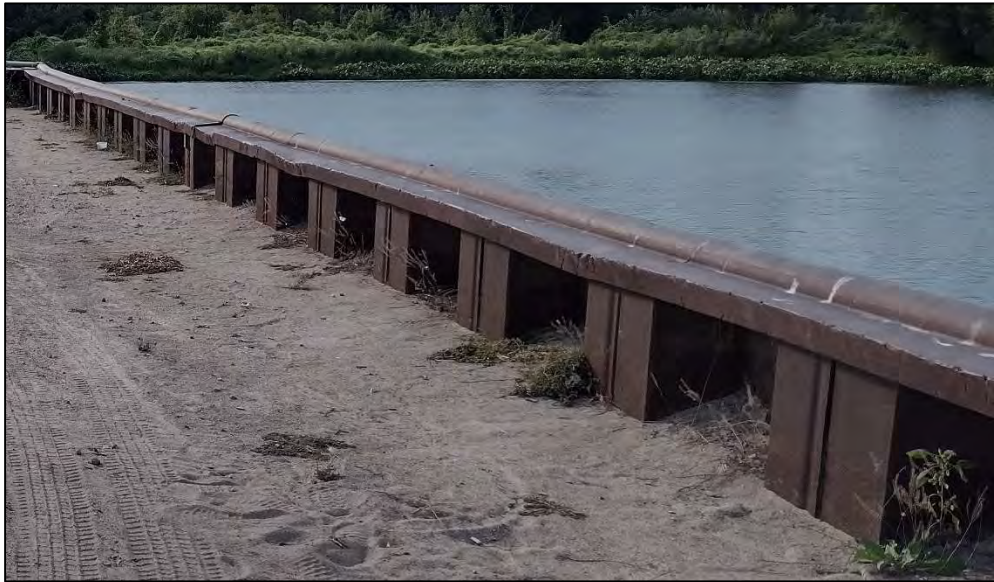
Figure 5: Miscellaneous Impact Damage to Dock Cap
