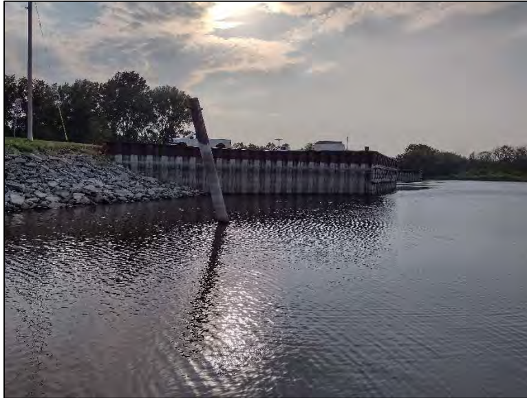
Figure 6: Current Condition of Single Mooring/Guide Pile
