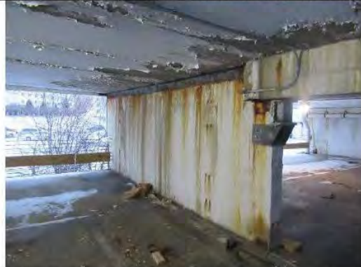
Photo 35: 7250 Parking ramp deterioration at bearing wall and steel angles and plates added to support deck above
