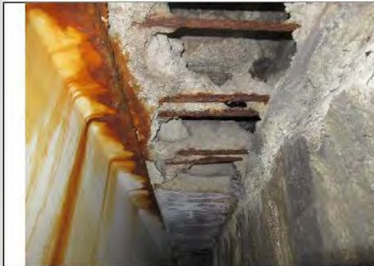
Photo 33: 7250 Parking ramp deteriorated precast concrete
